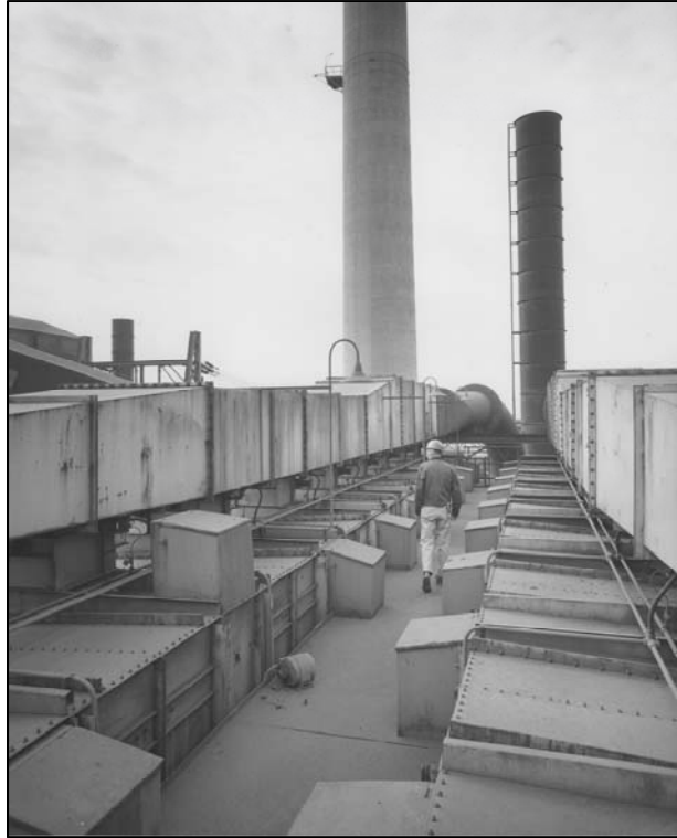
Figure 50. Environmental ductwork between furnace and sinter plants. 147
