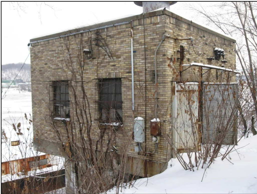
Photo 35. Pump House No. 1 (SC-26), front (southeast) façade and southwest elevation, view north
