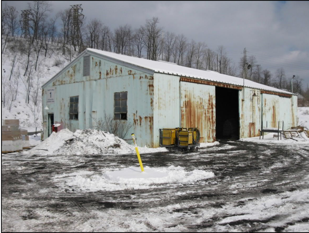
Photo 34. Power Plant Storeroom (SC-25), front (southwest) façade and northwest elevation, view east
