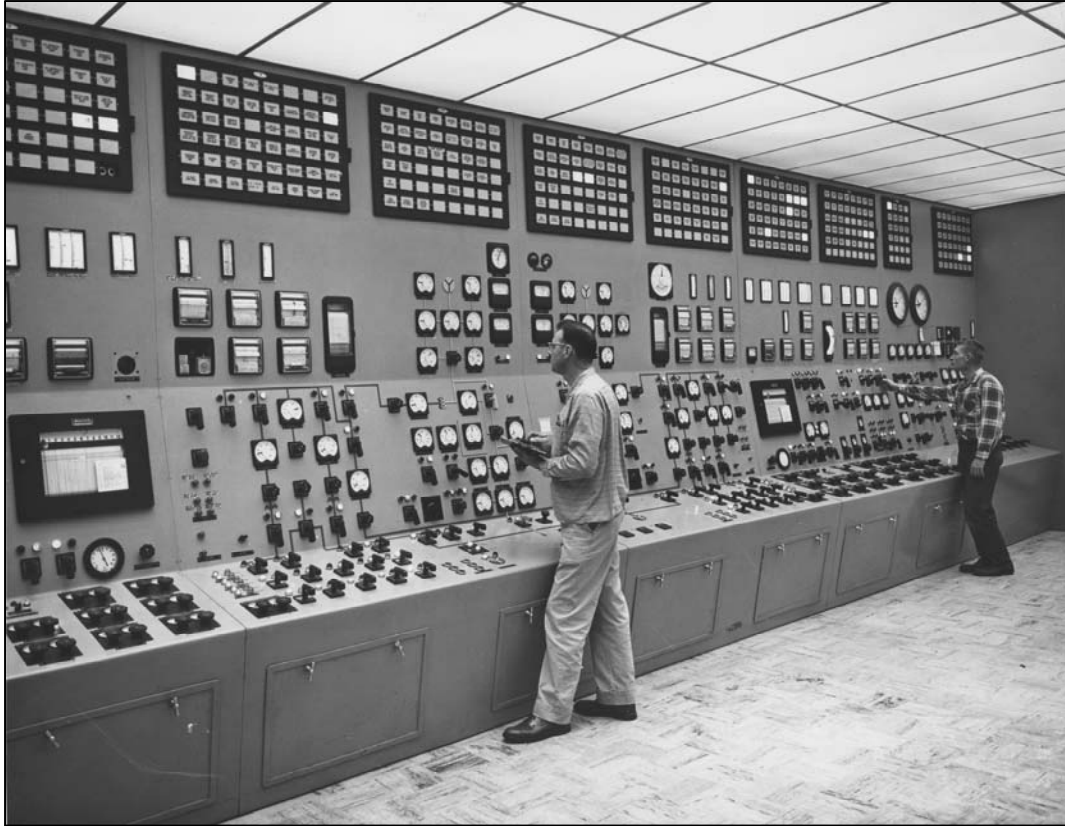
Figure 47. Power plant controls. 134
