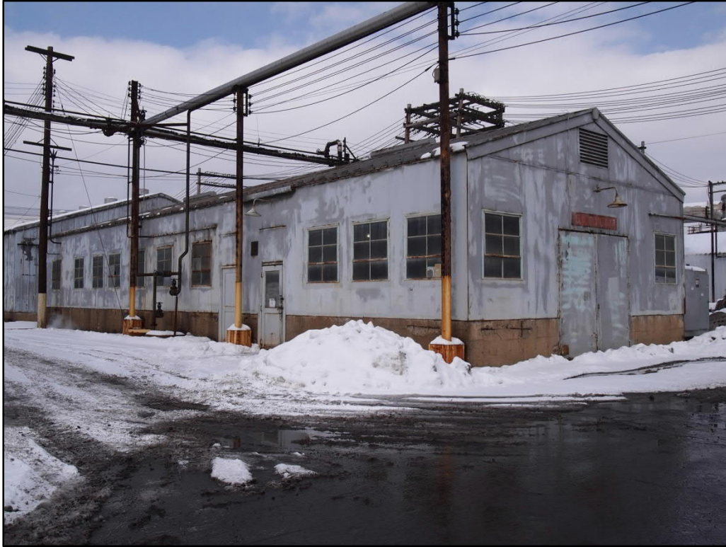
Photo 10. Electrical Maintenance Building (SC-8), front (southeast) façade and southwest elevation, view north
