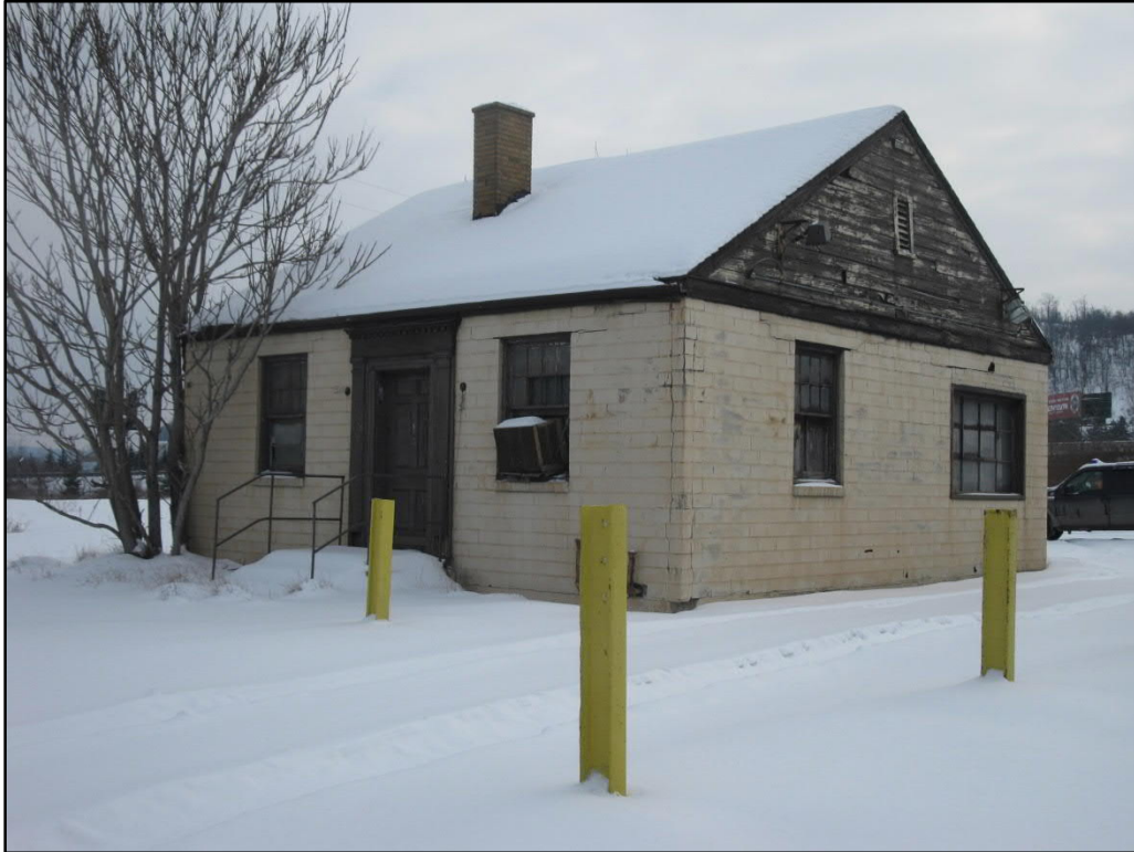
Photo 44. Truck Scale Building (SC-32), front (north) façade and west elevation, view southeast
