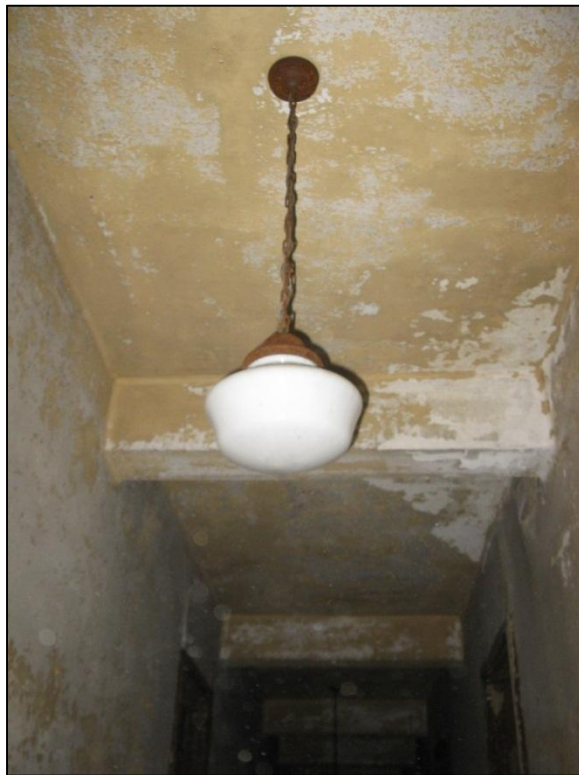
38. Beaver County Home. View of standard hanging light fixture.
