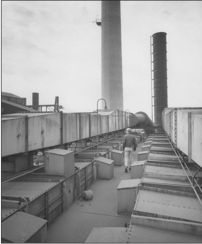
Figure 31. Environmental ductwork between furnace and sinter plants.
